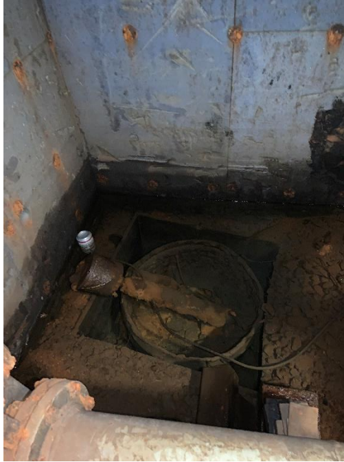
Photo 2.1.5: Sump pump and pit
