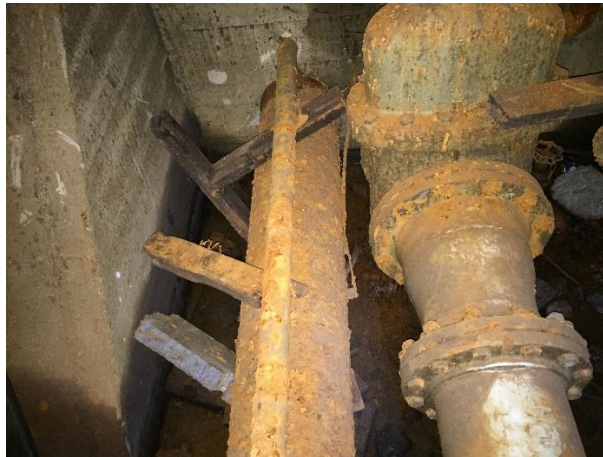
Photo 2.1.4: example of scrap metal propping up piping
