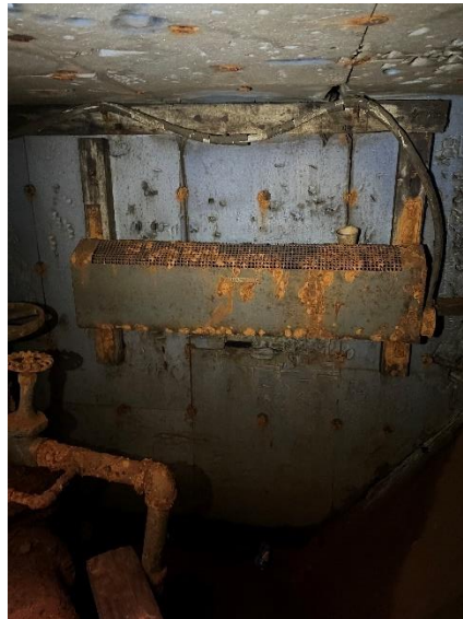
Photo 2.2.1: existing electrical radiant heater
